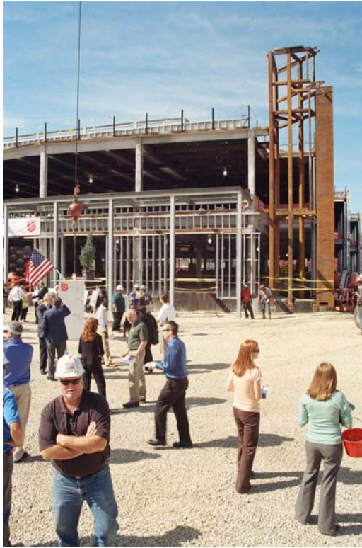
View of steel framing at the beacon at the northeast corner of the site.
